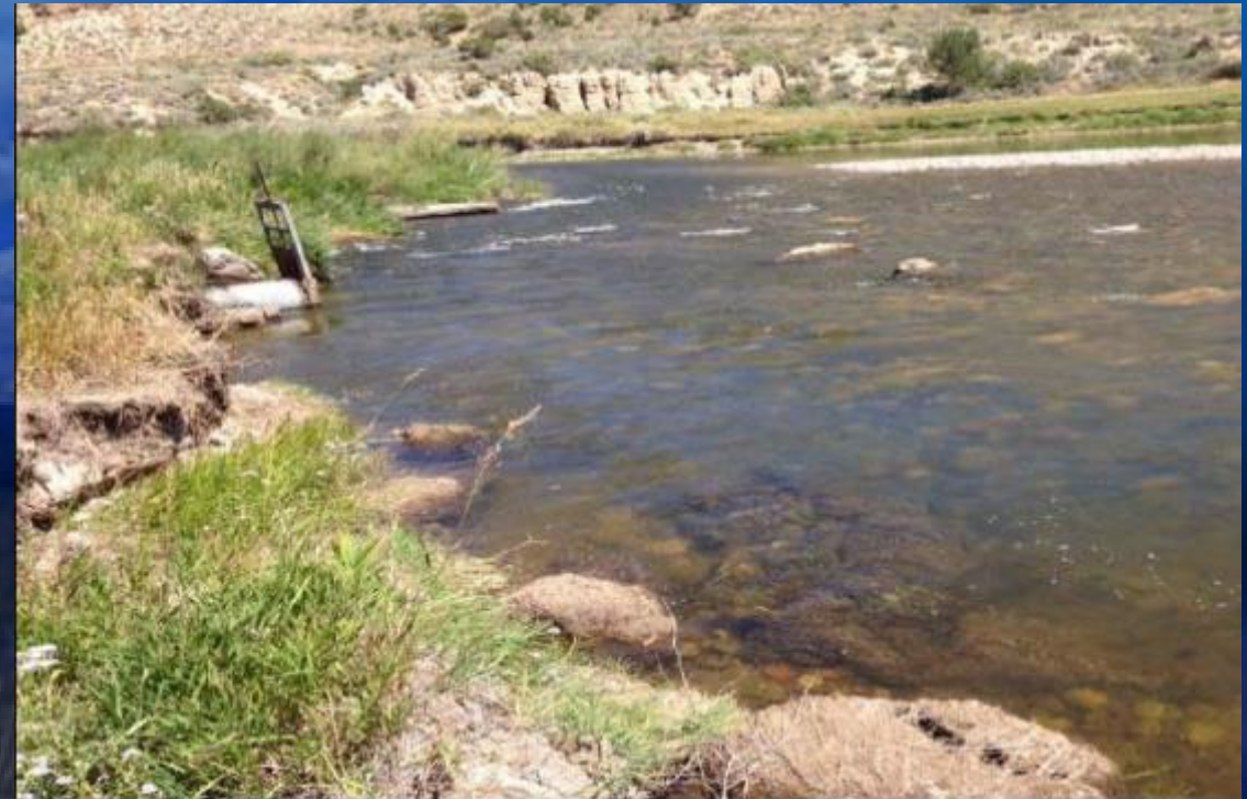
Before – Bank erosion, non-functional diversion and headgate
